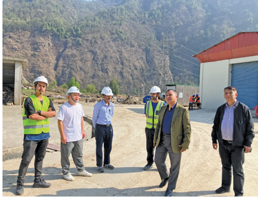
NEA Managing Director Kul Man Ghising and Deputy Managing Director Pradeep Kumar Thike and officials observing construction area of Markichowk-New Bharatpur transmission line.
